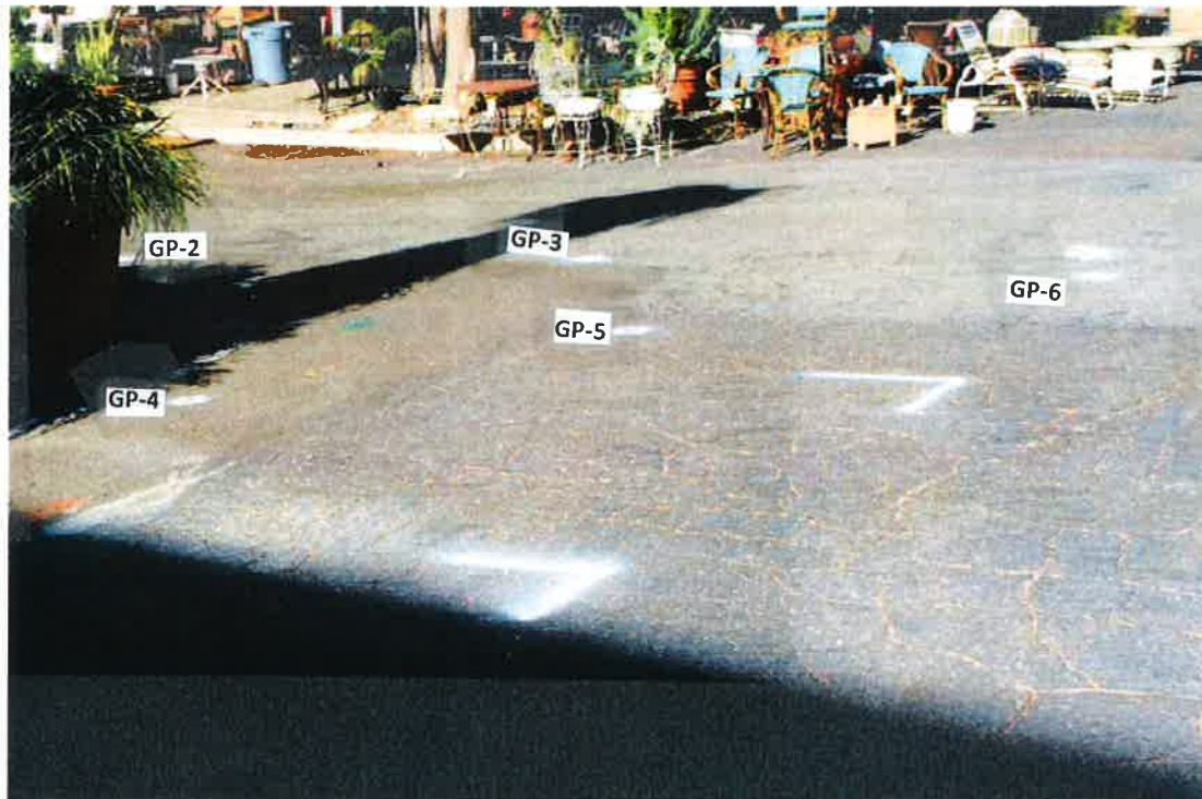
PHOTOGRAPH 2 – View looking west at the location of Boring GP-4 and the other Borings. The patio furniture on display across the parking lot is on the adjacent property at 400 West Coast Highway. The geophysical survey covered all the asphalt parking lot seen in the view and continued south along the driveway seen in Photograph 1.
